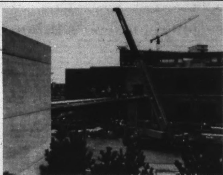
A skywalk between the Hotel and Conference Center is now under construction at the site north of Cavanaugh Hall. A skywalk is also being built between the Conference Center
