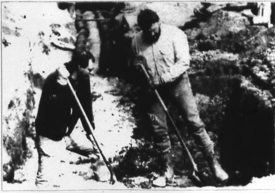
Warren Parman (left) and Curt Brinkmann break through rock and dirt to install part of a new heating and cooling system that is expected to bring heat in the winter and air conditioning in the summer to Cavanaugh Hall and other campus buildings.
