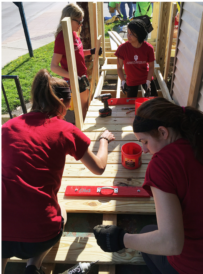
First-year OT students build a wheelchair ramp to improve access to the home.
