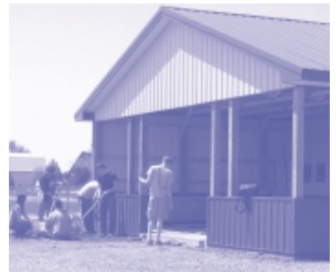
Pettisville agricultural science students conduct some final grading by hand of the area in front of the new addition.
