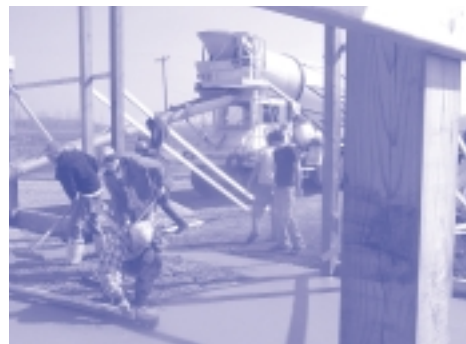
Pettisville agricultural business students help workers from two local businesses pour the concrete floor for the new extension. The concrete was donated. The company that directed the pouring provided discounts on the materials.
